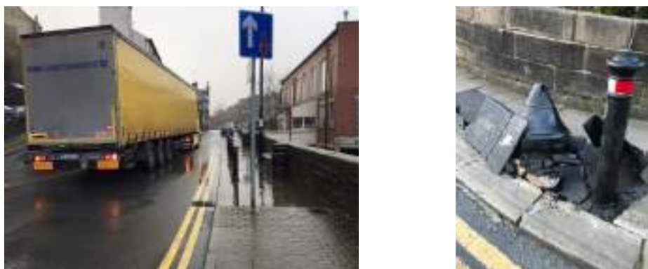
Figure 32 - Truck stuck on Hollowgate, Holmfirth & HGV damage to 'bell' protecting bridge on Hollowgate
