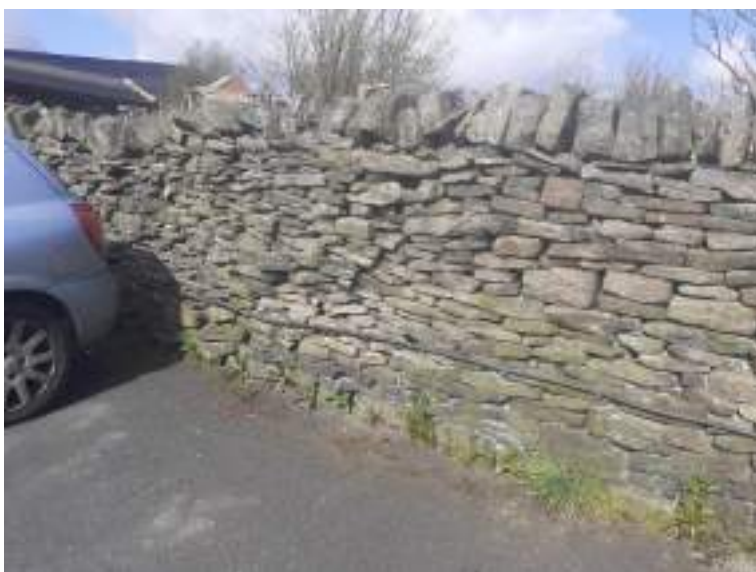
View 5 – Slightly damaged wall at back of car park
