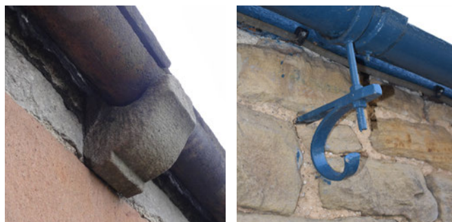
Left: Stone support for a cast iron gutter on a historic barn. (© Oldfield Design Ltd). Right: Metal bracket gutter support on a former smithy. (© PDNPA)
