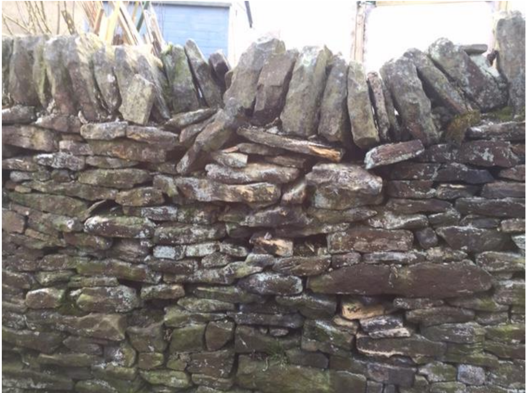
Disrepair of Watery Lane Allotments Wall
