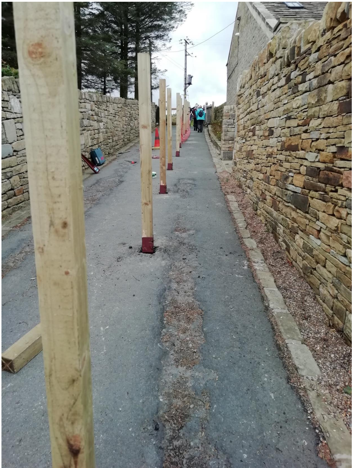
Photos of work being undertaken to the Public Right of Way at Wolfstones Farm:
